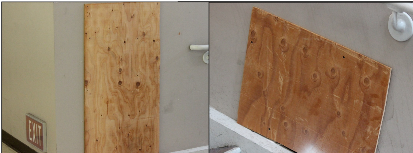
Two of five holes in the A Building stairwell are covered by plywood.
